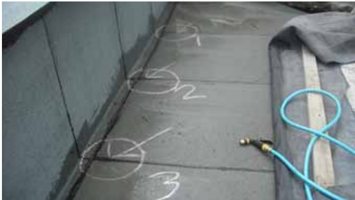
Breaches in Torch-on Membrane
